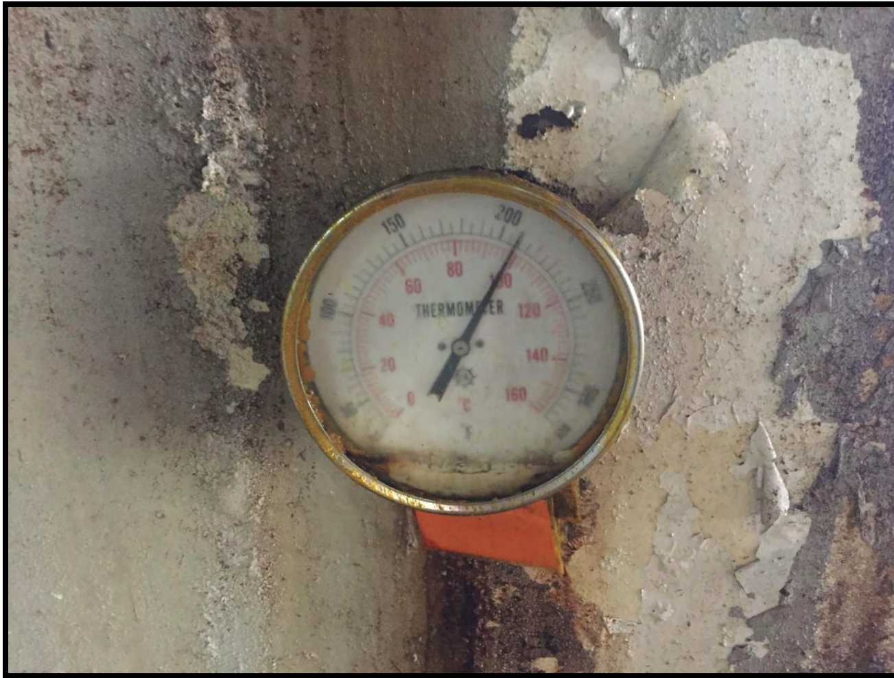
CRUDE OIL TANK
