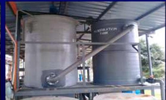
Chemical and polymer mixing tank
